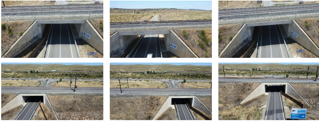
Figure 19: Sample of images extracted by the recording referred to the Underpass Bridge in Demo Site #1.
