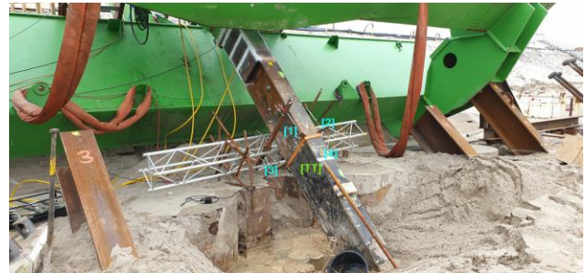
Fig. 7: Reaction frame, test pile in the centre, left reaction pile not visible, right reaction pile on the right in the picture.
