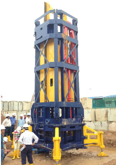
Figure 2. StatRapid System for Rapid Load Testing of Piles at Punggol C36 Project
