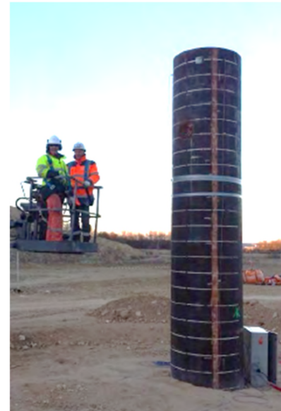
Fig. 1. Test setup with accelerometers and manually applied hammer stroke from a cherry picker
