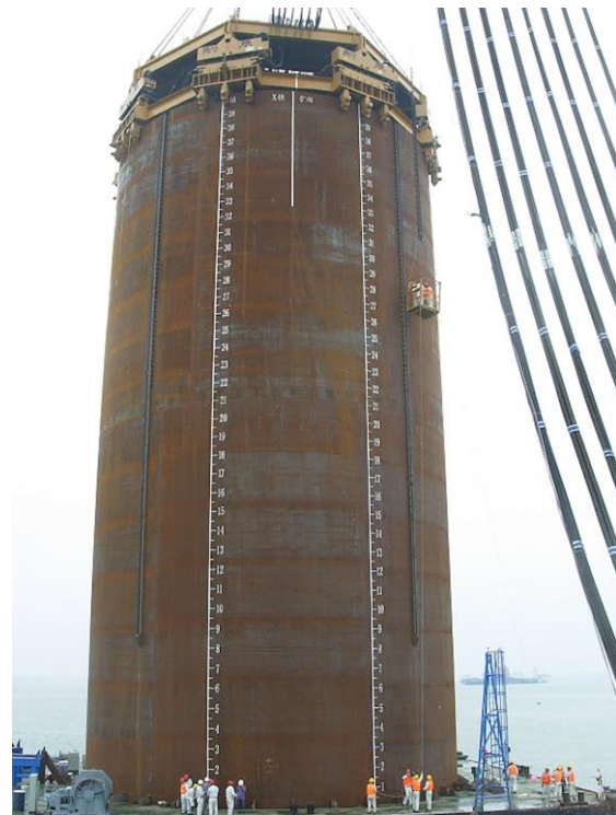
Fig. 32. Vibratory driving of a 22m diameter caisson for the Hong Kong-Zhuhai-Macau Bridge project
