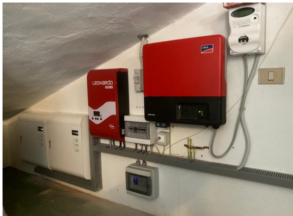
Figure 59: 09_Home battery installed
