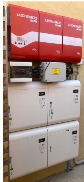
Figure 62: 38_Home battery installed
