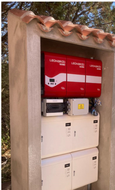
Figure 61: 04_Hotel battery installed
