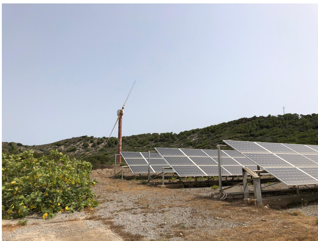
Figure 33 NASCA PV Plant of 1MWp
