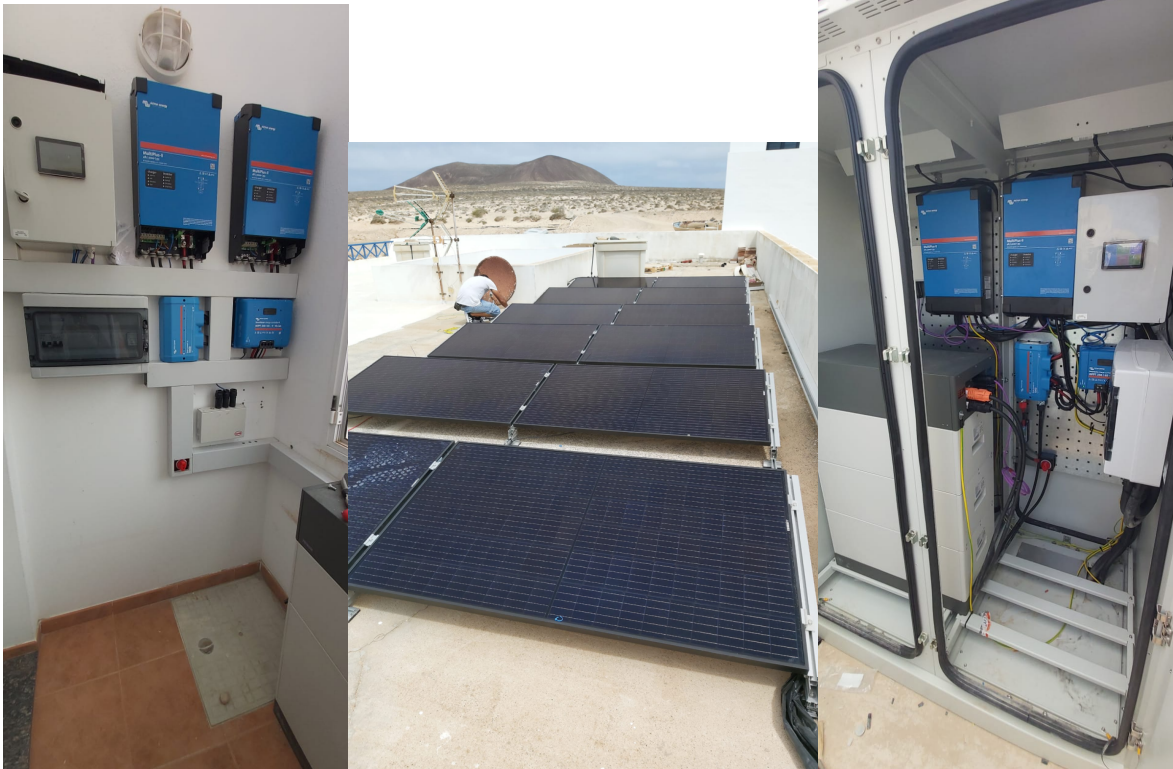
Figure 56 installations in buildings with scenario type 4
