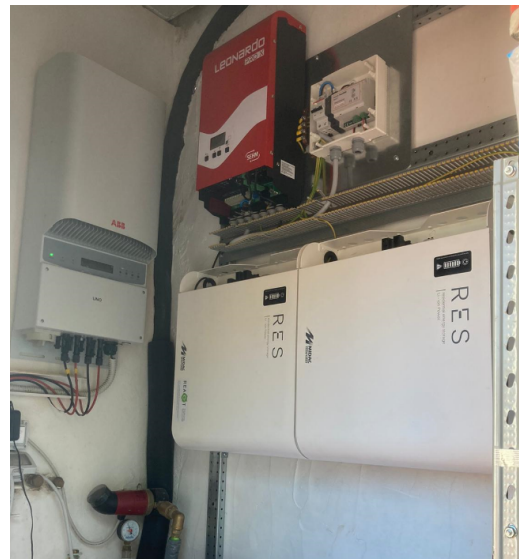
Figure 60: 33_Home battery installed
