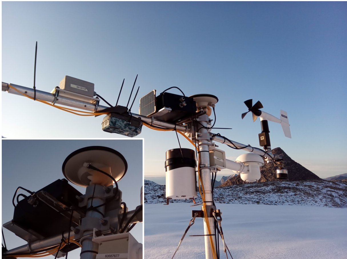
Figure 2.1.4. The INTAROS high accuracy GNSS instrument and power supply are contained in the black anodized aluminum enclosure mounted on the instrument boom of the NUK-K PROMICE AWS. The Novatel Pinwheel antenna and the 2 W solar panel are also visible.
