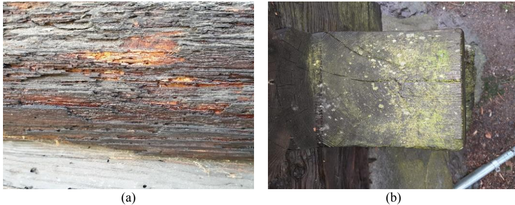
Figure 5: Biological defects in Heierstad Loft
