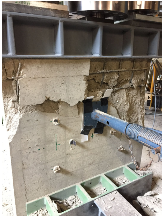
Figure 21: Reinforced wall failure
