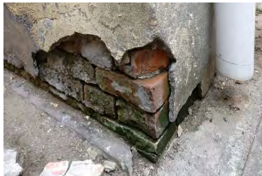
Figure 11 The brick foundation is eroded. (Image source: photographed by the author)
