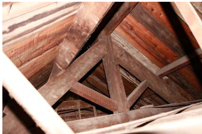
Figure 21 Roof truss of building No.2 before conservation (Image source: photographed by the author)
