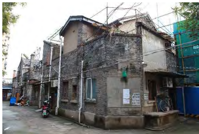
Figure 13 The exposed pipes have influenced the historical features of the buildings. (Image source: photographed by the author)
