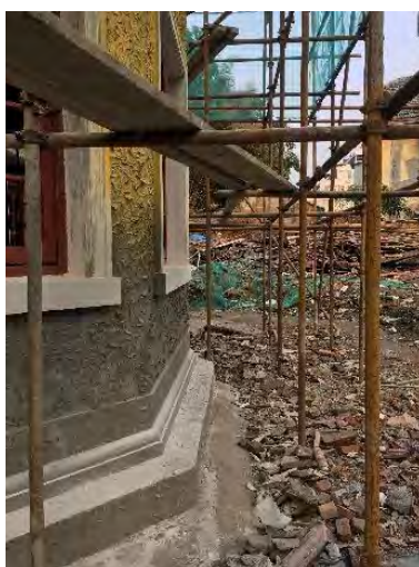
Figure 14 The building foundation that has been reinforced. (Image source : photographed by the author)
