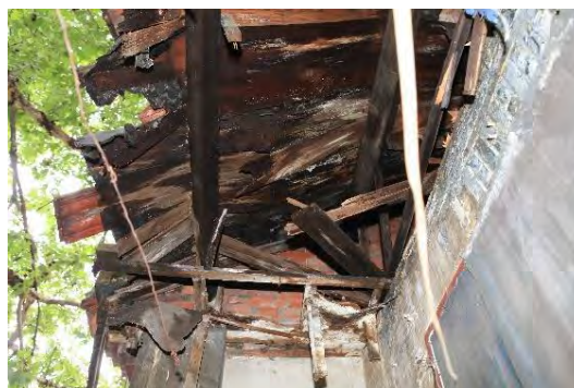
Figure 12 The roof of some buildings leaked r. (Image source: photographed by the author)
