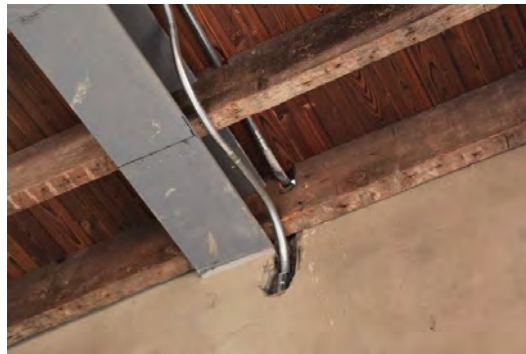
Figure 20 The steel beam is placed inside the wall and bonded with cement mortar (Image source: photographed by the author)
