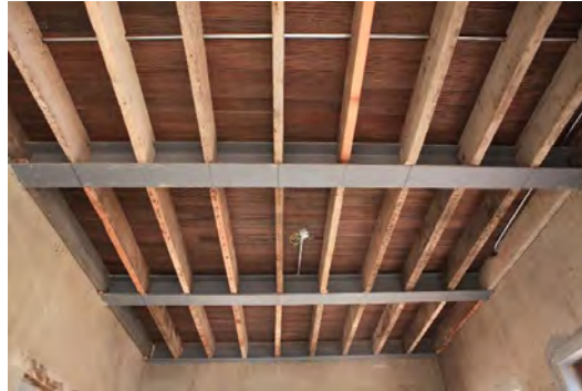
Figure 19 Replaced the original wooden beams with I-beams (Image source: photographed by the author)
