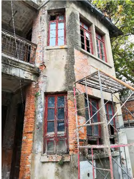
Figure 17 Carefully peeled off the cement mortar and restored the historical appearance (Building No. 2, image source: photographed by the author)
