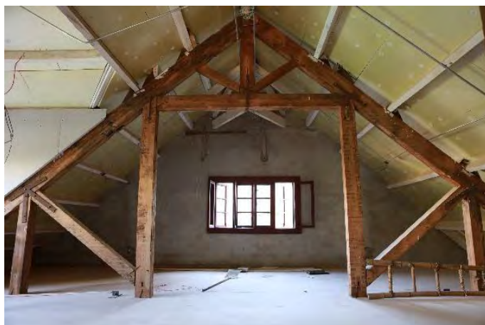
Figure 22 Wooden roof truss system of building No.2 during conservation (Image source: photographed by the author)
