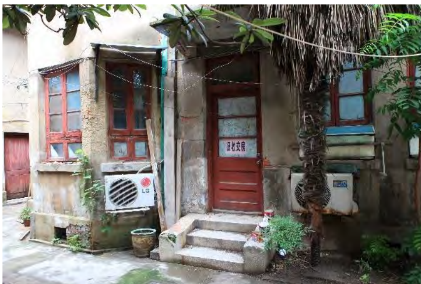
Figure 23 Residents installed a lot of air conditioners before conservation (Building No. 2, image source: photographed by the author)
