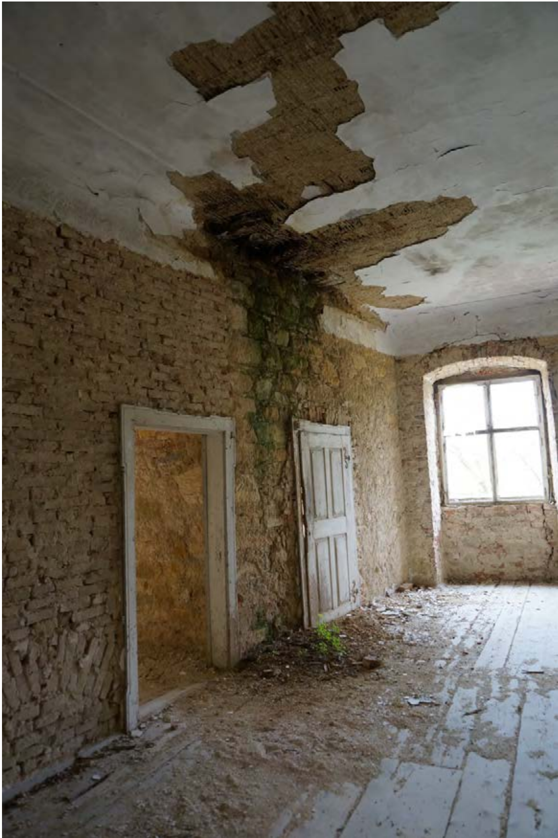
Figure 22. Biological cause, damaged roof, lack of maintenance
