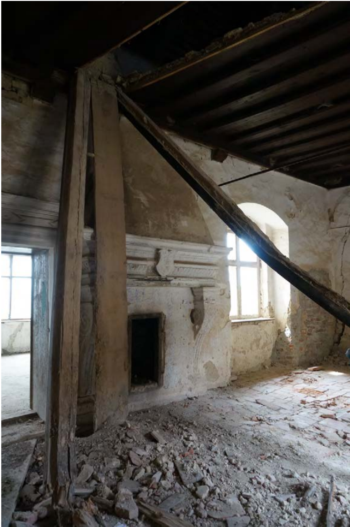
Figure 21. Collapse of the Renaissance wooden ceiling due to lack of maintenance
