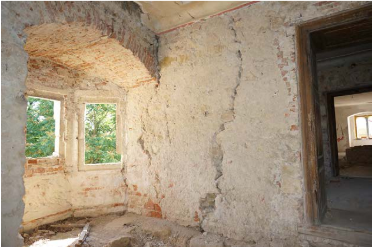
Figure 14. Man-made cause, destructive research method, removal of floor surfaces, vertical cracks
