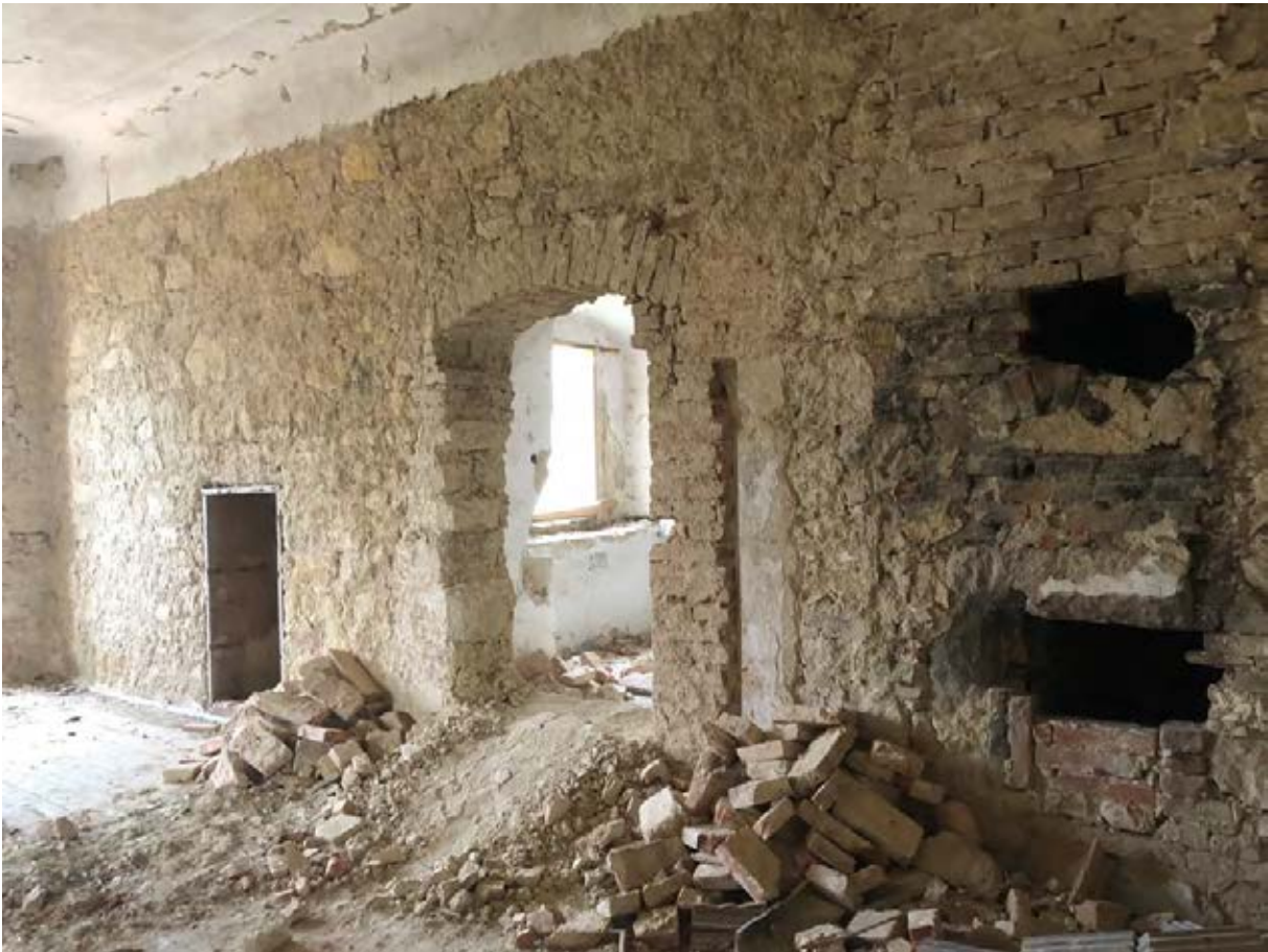
Figure 16. Man-made cause, destructive research method, recent (2017) opening of historic doors and windows
