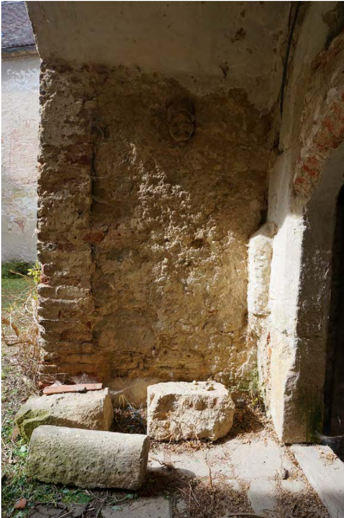
Figure 20. Stone elements (spolias) exposed to weathering
