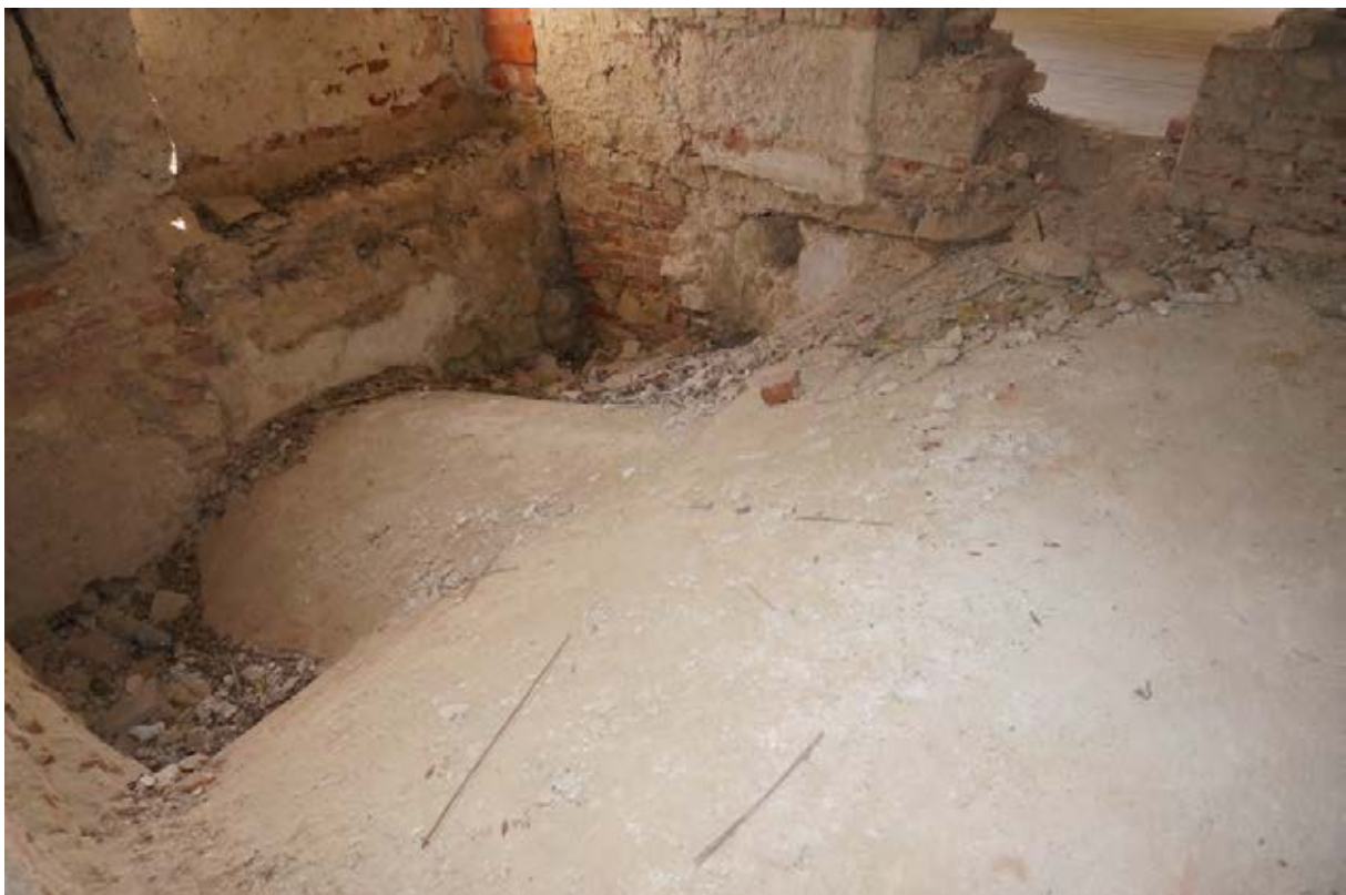
Figure 15. Man-made cause, destructive research method, removal of floor surfaces since 2006
