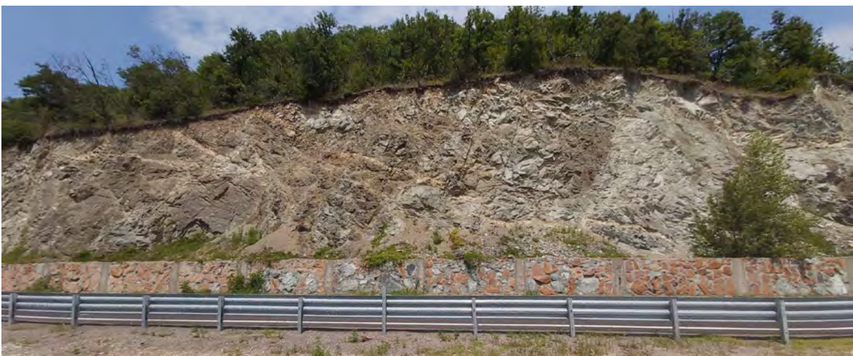
Fig. 25 The Luți gabbro with faulted intrusions of plagiogranite, in a spectacular outcrop upstream of Luți valley, Iron Gates Gorges, the metamorphic basement of the Danubian Units
