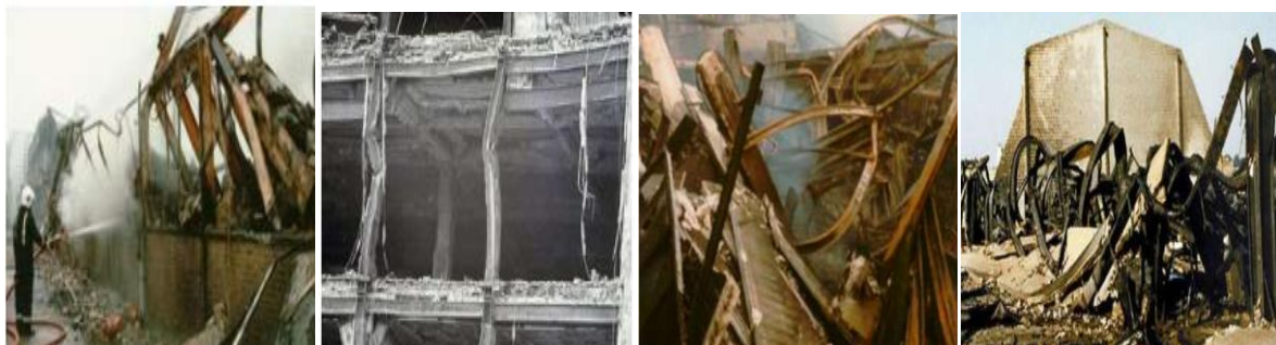
Fig. 1: Deflection of Structural Steel after a fire and Structural Steel has collapsed after a fire
