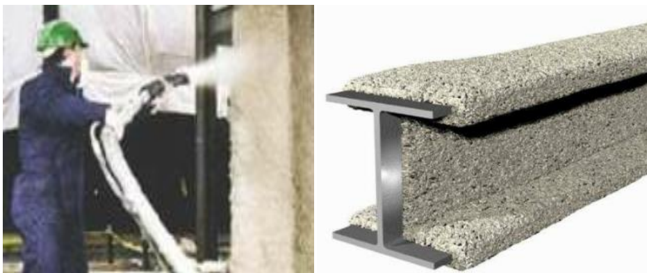
Fig. 7: Illustration of the procedure for spraying wet spray vermiculate cementitious and the results
