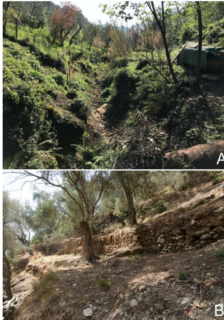
Figure 4. Terraces in the case study area: (A) not maintained in Paraggi catchment (n. 8 in Figure 1) close to the stream, and (B) partially maintained in San Fruttuoso (Figure 1, catchment n. 3).
