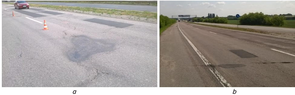
Fig. 4. Results of visual inspection of the road section (example): a – a grid of cracks with pit repairs; b – transverse cracks
