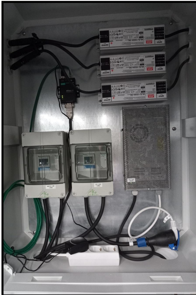
Figure 4. Regulation utility box housing our two timers, three power supplies for the Osram RLs, our MOXA port, the HE 24-V LED power supply, and green network cable connecting to our router for remote control.
