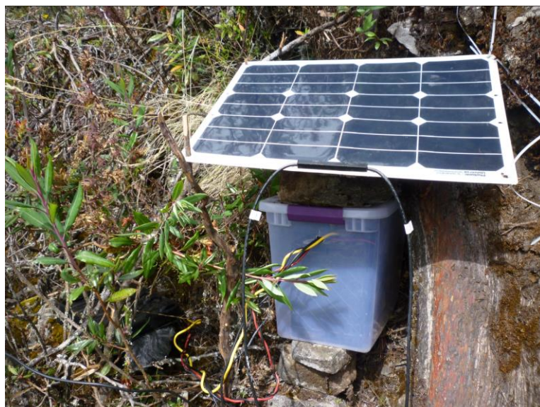
Figure 3. Streambox, battery housing and solar panel in initial installation position in
