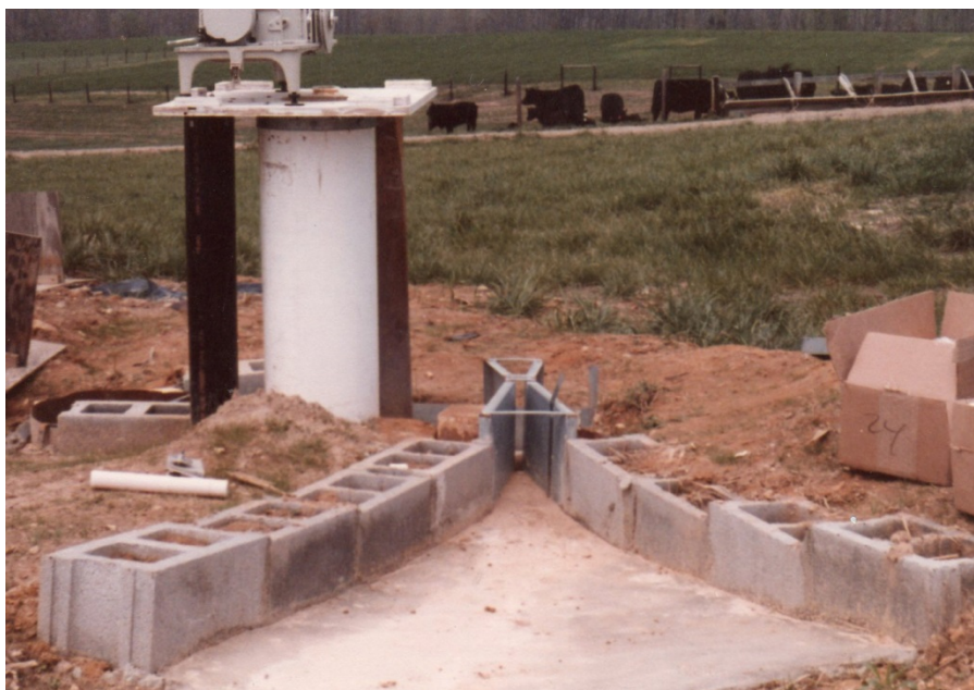
Figure 3-4. Field application of small Parshall flume
