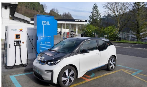
Figure 58: Buffer battery for fast charger in Spain with recycled EV batteries
