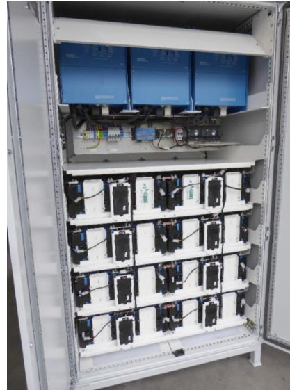
Figure 56: Watt4Ever 40kWh battery for the storage of PV energy
