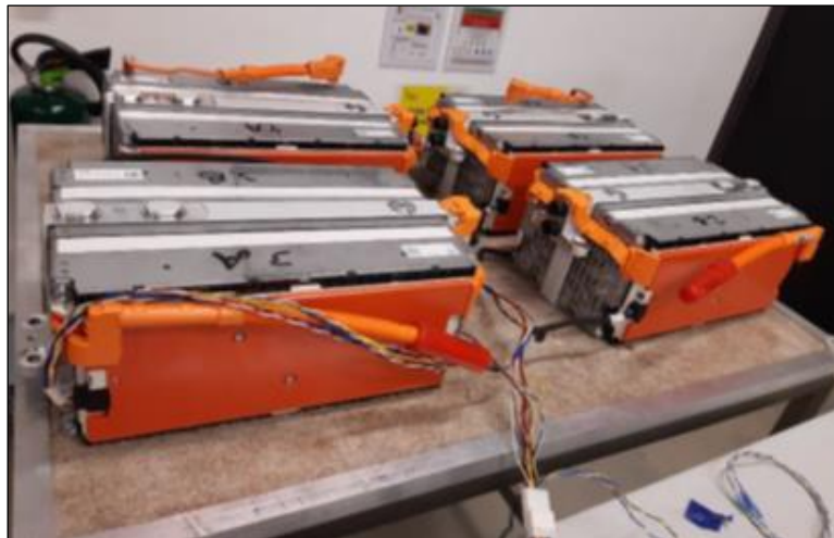
Figure 45 – Battery modules taken out of the pack's casing with direct measurement of cells' voltages
