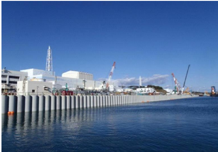
Fig. 6.4. Picture of the seaside wall (after TEPCO HP). This wall cut the groundwater discharge from the main two aquifers in Fig. 6.2.
