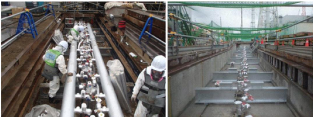
Fig. 6.5. Ice wall construction, over than 30 m length freezing pipes were settled by every 1.0 m on the mountain side and 1.2 m on the seaside (after TEPCO HP)
