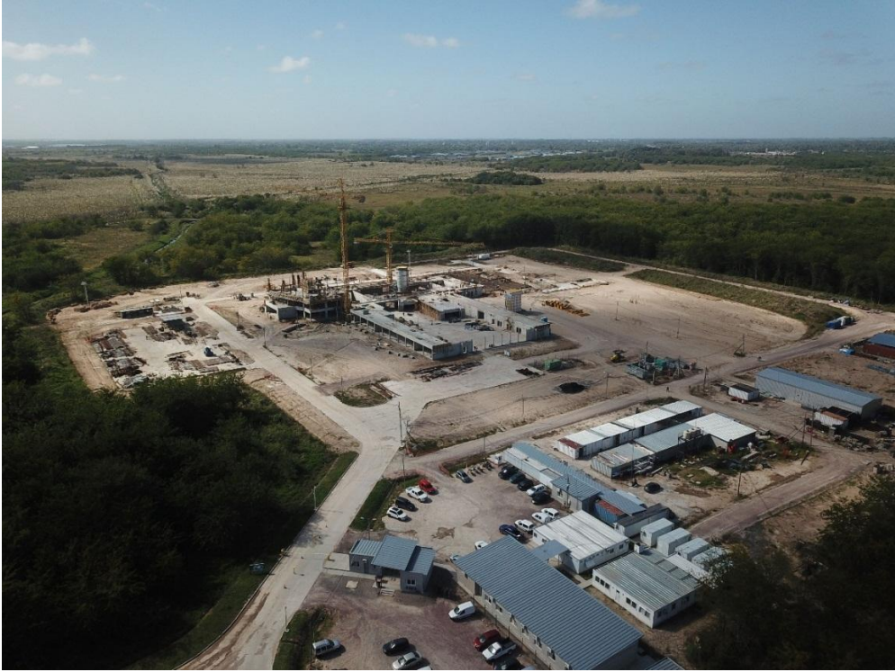
Construction site of the RA10 reactor in the Ezeiza Atomic Center https://www.argentina.gob.ar/cnea/ra10/en-imagenes.
