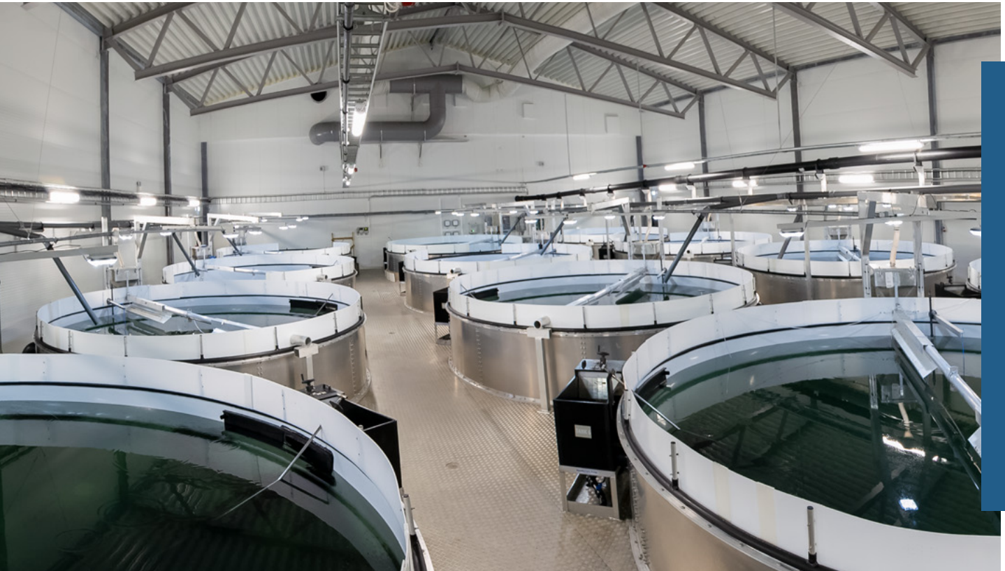
Recirculation Aquaculture System - Norway
