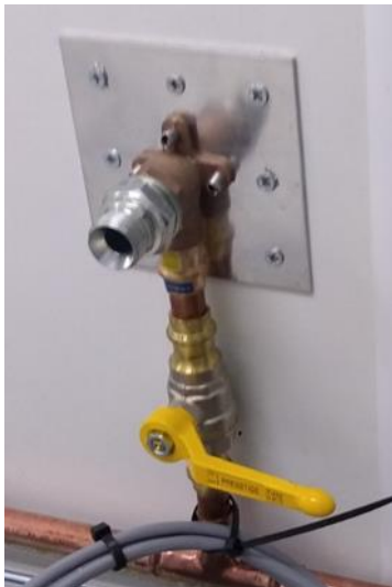
Figure 10 Gas valve with opening for outflow
