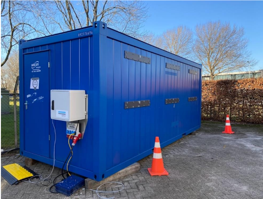
Figure 11 Photo of side of the container with the 6 vents
