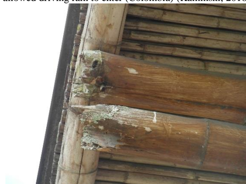
d) Rotten bamboo where a beam was exposed and collected water (Costa Rica) (Kaminski, 2016)
