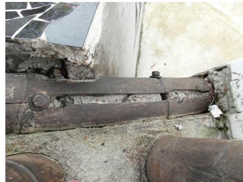
b) Rotten bamboo chord of a bridge, where a bolt hole allowed driving rain to enter (Colombia) (Kaminski, 2016)
