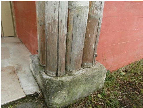
a) Rotten bamboo columns which were exposed to driving rain (Colombia) (Kaminski, 2016)
