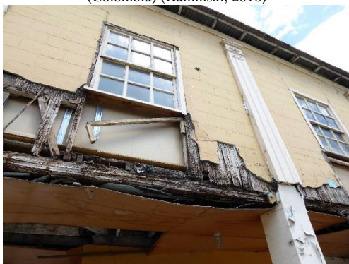
c) Rotten timber and bamboo inside the wall (Ecuador) (Kaminski, 2016)
