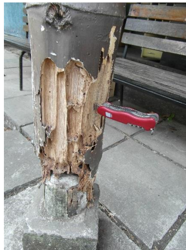
b) Significant termite damage to bamboo column (Costa Rica) (Kaminski, 2016)
