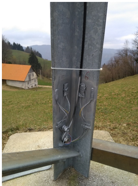
Fig. 2. Adhesive strain gauges at the location of the measured residual stresses on the L profile of the SW foot
