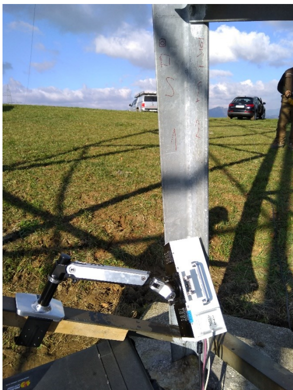
Fig. 1. Measurement of residual stresses on the NE leg at the 1st measuring point
