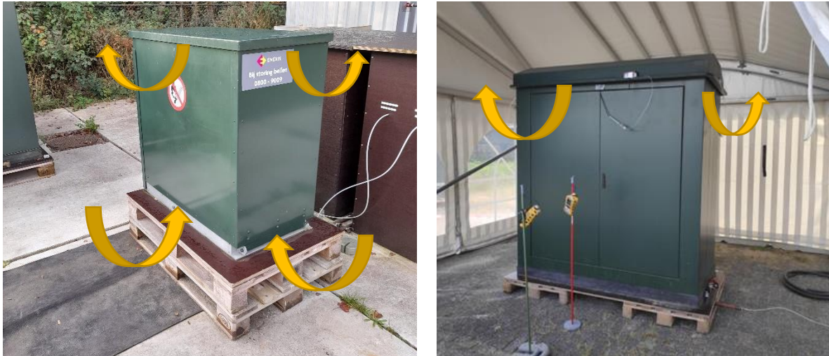
Figure 15. Small cabinet ( \frac{1}{2} m 3 cabinet) on left and large cabinet (4 m 3 cabinet station) on right
