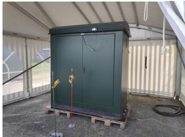
Figure 6. The 4 m 3 cabinet station in a tent
