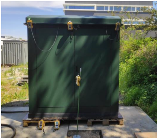
Figure 24. The 4 m 3 cabinet station in an outdoor situation
