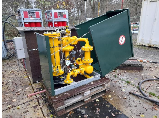
Figure 23. The 1/2 m 3 cabinet containing the gas pressure
