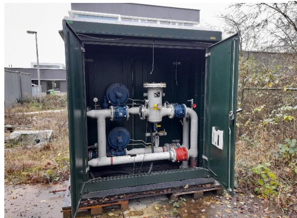
Figure 25. The 4 m 3 cabinet station containing the gas pressure reducing station
