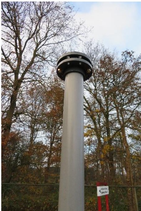
Gas filter and vent 2
