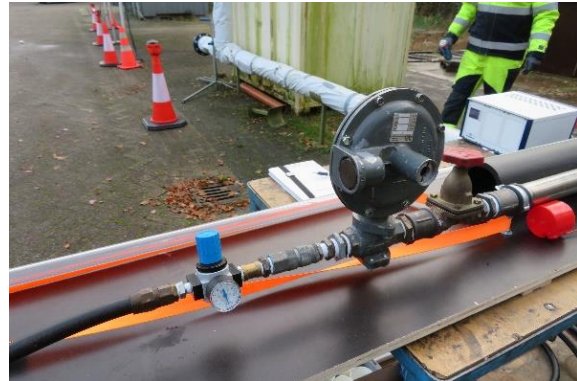
Control valve and pressure reducing valve
