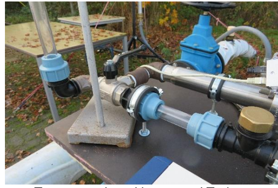
Two-way valve with vent and T-piece
