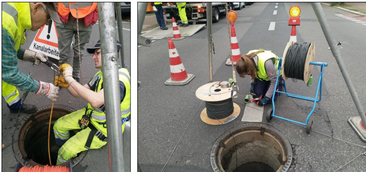
Figure 13: Storm sewer manhole located in the middle of the street (right); preparations to realize access to the sewer system via house connection (left).
