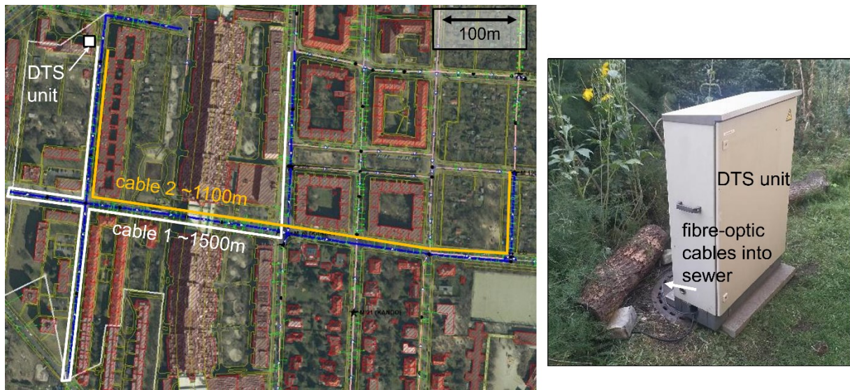
Figure 11: Overview of studied sewer system and fiber-optic cable routes (left); DTS unit installed at Bezirksamt Charlottenburg (right)
