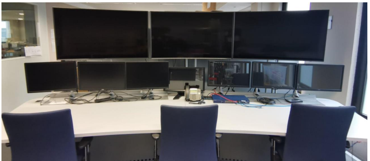
Figure 31. Remote control centre setup prepared for running the SCC
