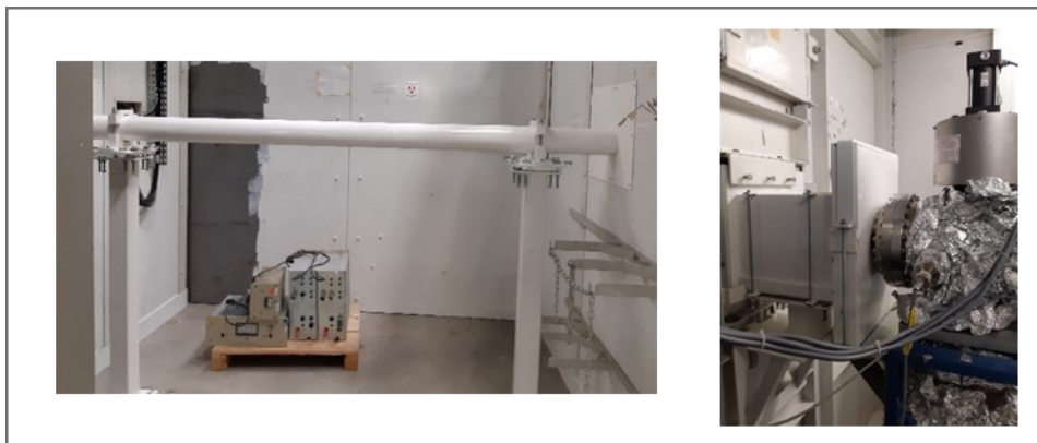
Figure 1: Left: a new slim shielding for the connecting tube between EH1 and EH2. Right: the refurbished shielding after the main beam shutter in the Optic Hutch.
