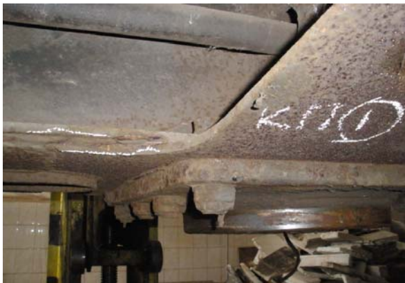
Fig. 5. The crack on the welding seam at the joint of the lower sheet of span bolster with the longitudinal tie rod
