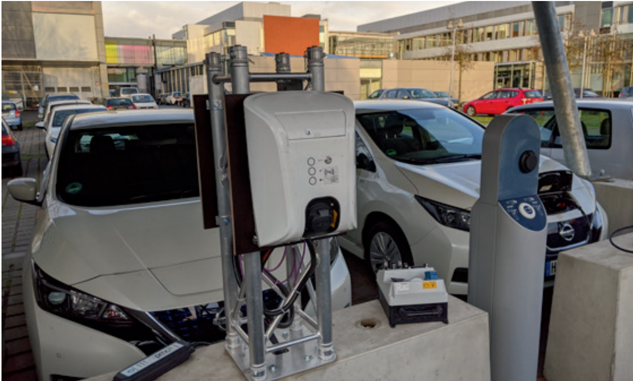
Figure 14: PMC solar carport with buffer storage and smart charging at the IFAM in Bremen, source: PMC
