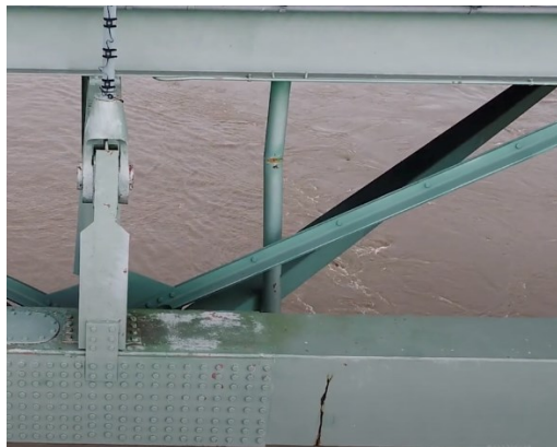
Figure 3.1: Drone footage from 2019 shows the crack already existed. (Photo courtesy of ARDOT via YouTube)
