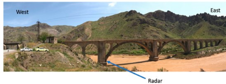
Figure 2.31. Analysis of the Kafan-Kuh bridge, Northern Iran using Ground-Based data (Pieraccini et al. 2019).
