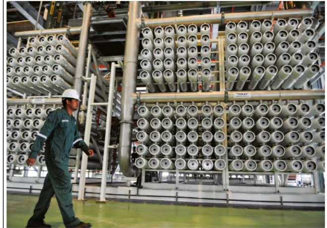
One of five water-reuse plants in Singapore, which together supply about 40% of the nation's water for drinking and other uses.
