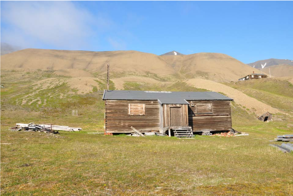
(6) Building B (telegraph, general store and provision storage) in Hiorthhamn, scale 2m, looking NE. (Photo: S. Dresscher, 2014.)
