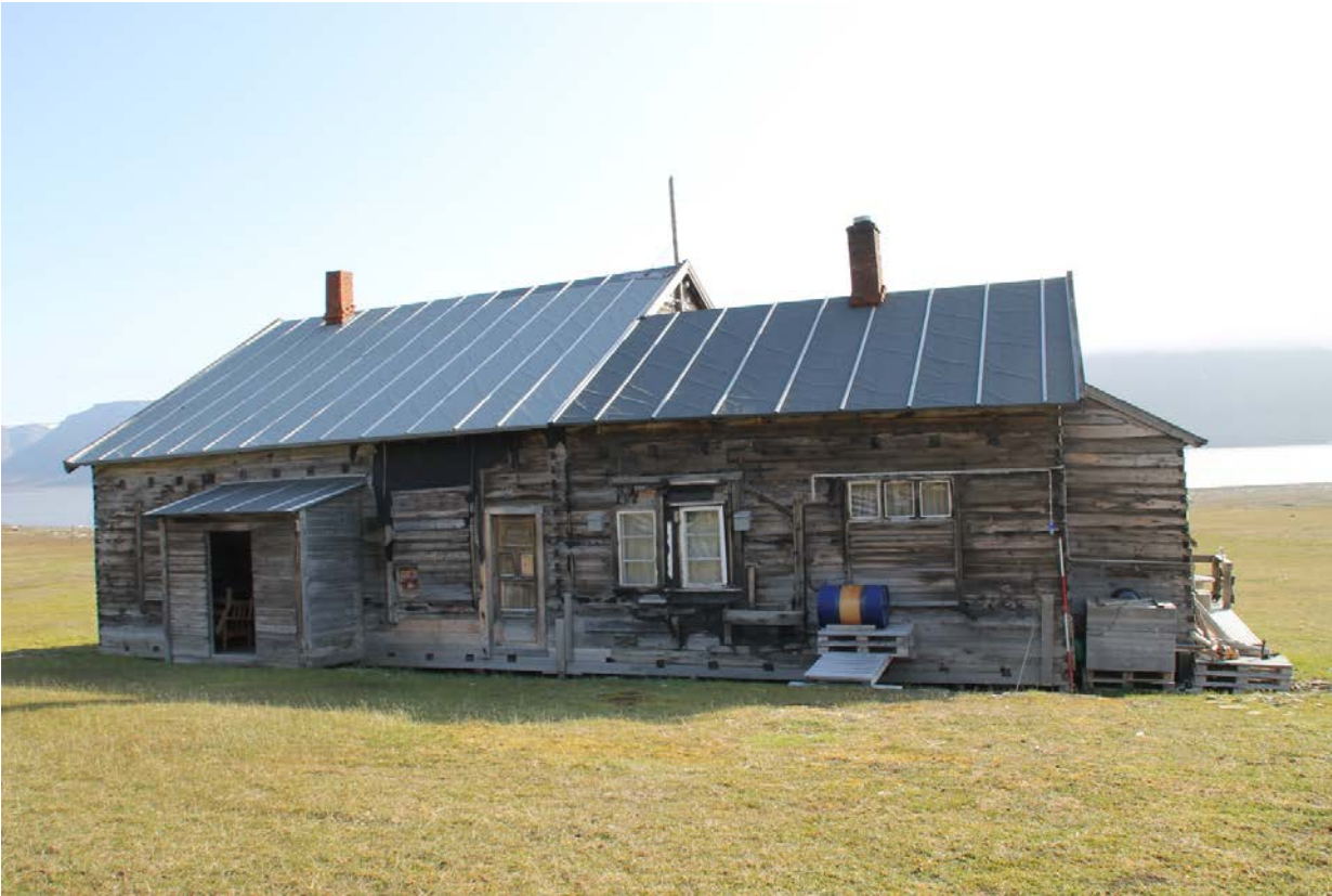
(6) Building C (living quarters) in Hiorthhamn, scale 2m, looking SW. (Photo: S. Dresscher, 2014.)
