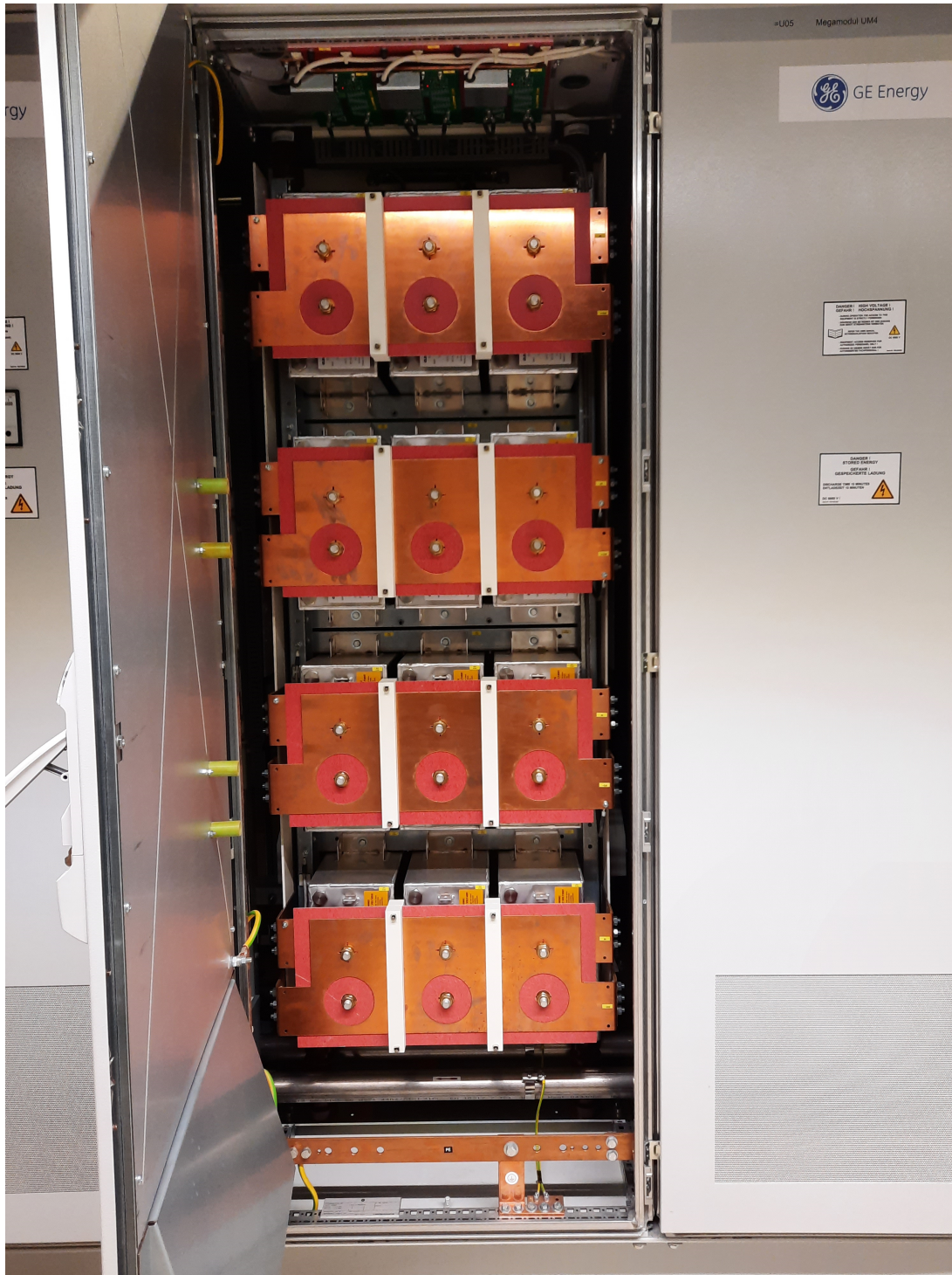
Figure 11: Capacitor banks of the converters of the FEN MVDC Research grid.
