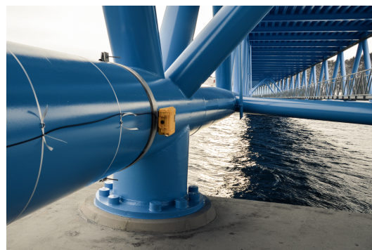
(e) Canterbury Seismic Instruments CUSP-3, triaxial accelerometer.
