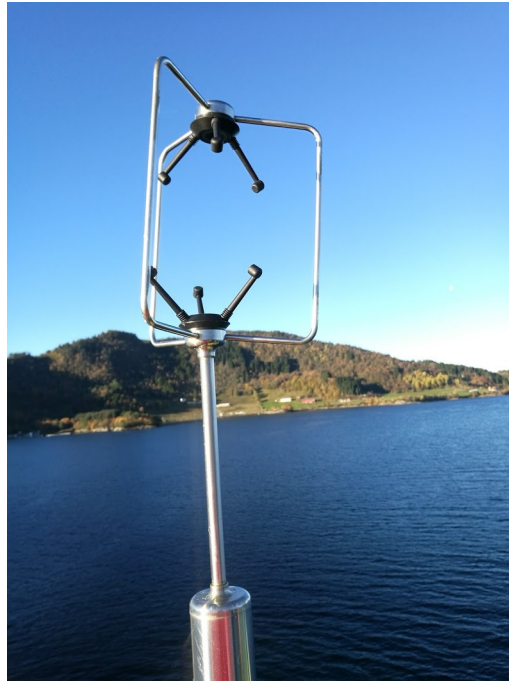
Figure 5. Damaged anemometer A3 needed to be changed during sensor layout revision Main .
