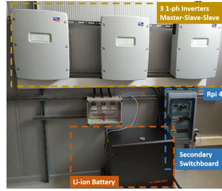
Fig. 4: BESS residential three-phase installation.
