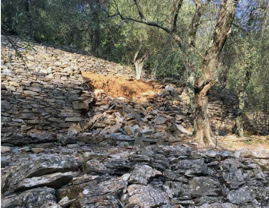
Fig.1 Dry-stone wall collapse in a terrace system of Liguria (P. Tarolli)
