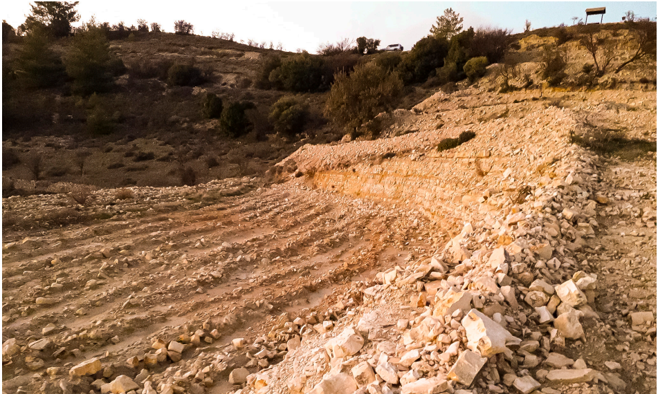
Figure 9. A close-up view of newly prepared vine terrace using subsidized mechanised means below Aeton Moutti hill, in contrast to traditional terracing seen in the background (photo by Sevina Floridou).
