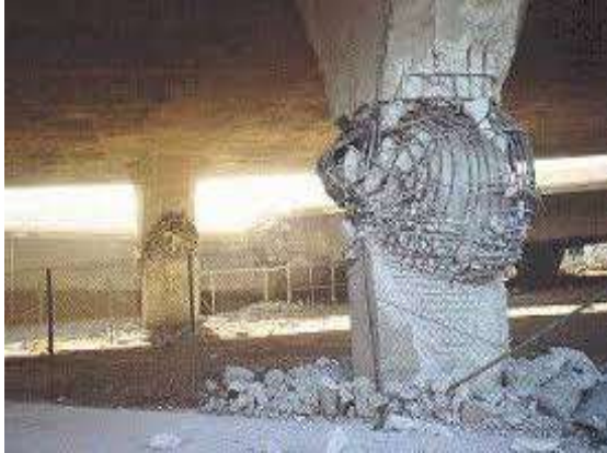
Fig. 4 Plastic deformation of a bridge concrete column
