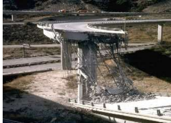
Fig. 5 A superstructure failure
