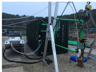
Figure 6: 400 kW Thermal Response Test (TRT) rig with "air blaster" – external and internal viewpoints.
