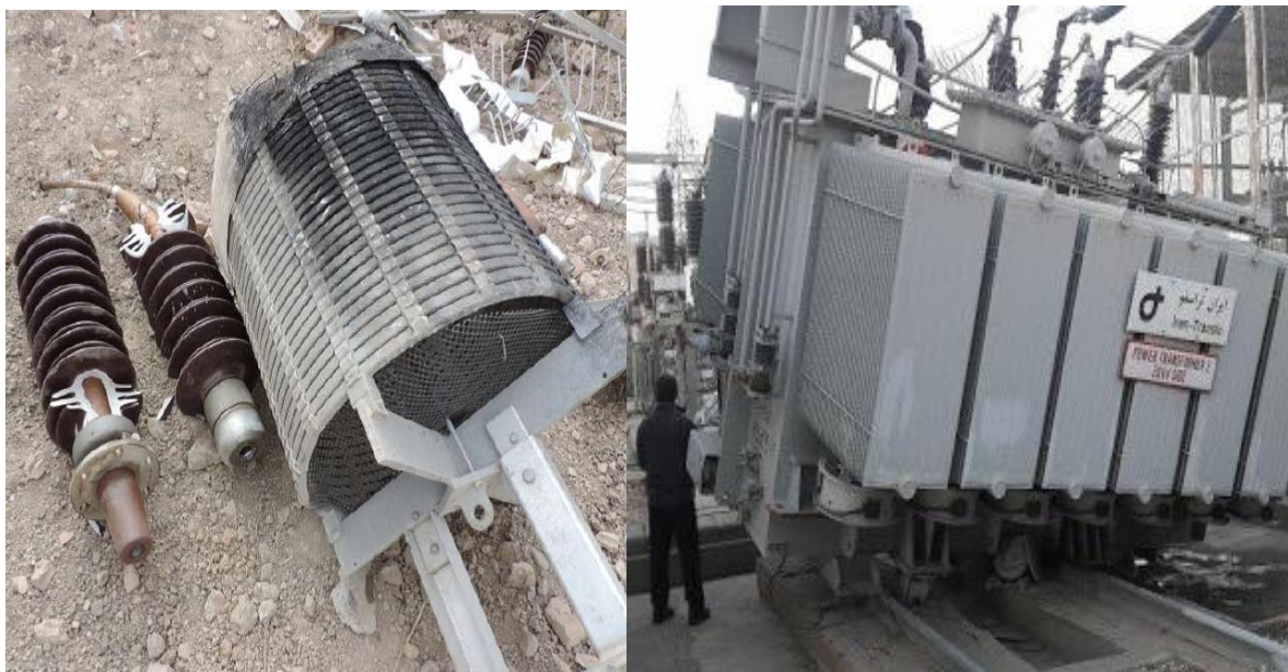
Figure 10. Damage in Substations (2017 Kermanshah Earthquake__Iran)
