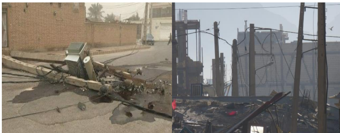
Figure 9. Damage in Distribution Circuits(2017 Kermanshah Earthquake __Iran)
