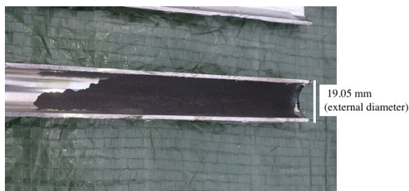
Figure 3- Example of a tube showing the black scales deposited on the internal metal surface.
