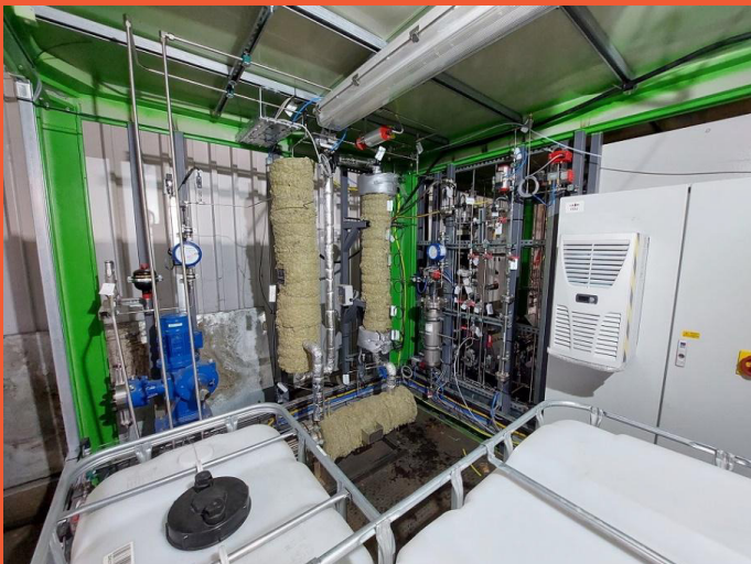
APR process demonstration unit (©BEST GmbH)
