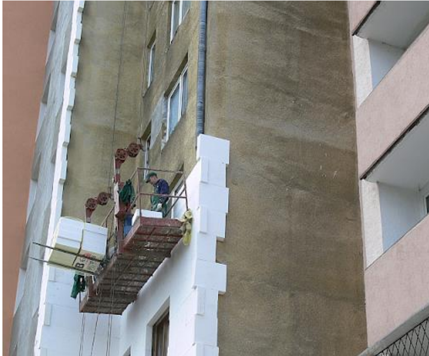
Fig. 17. The most popular method for wall thermal modernization in multi-family buildings in Poland.
