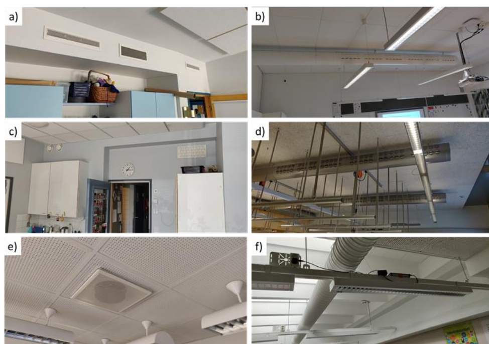
Figure 2. Typical air distribution methods in measured indoor environments: (a) wall air distribution of playroom in kindergarten 2; (b) duct air diffuser of classroom in primary school 1; (c) wall air distribution of playroom in kindergarten 3; (d) duct diffuser of classroom in primary school 4; (e) ceiling air distribution of classroom in primary school 2; (f) duct diffuser of classroom in secondary school.
