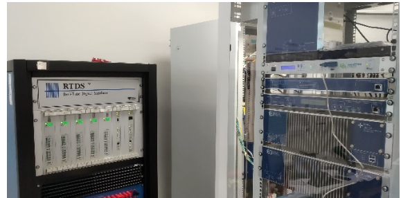
Figure 3. View of the RTDS connected to the equipment
