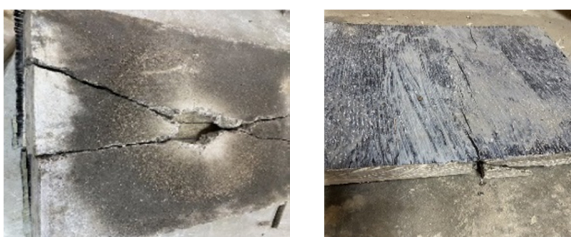
Fig. 5. Typical failure behavior of reinforced concrete slabs.
