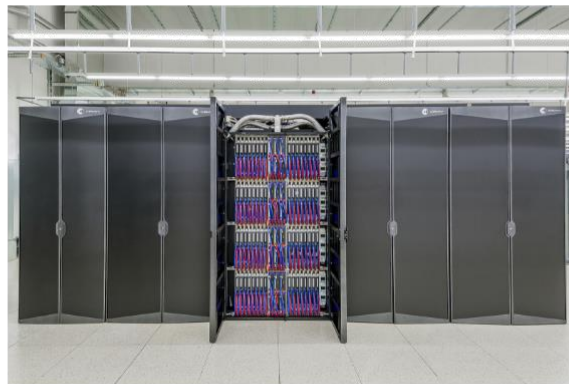
The first cabinets of the “Alps” research infrastructure have been installed in November 2020. (Image: CSCS)
