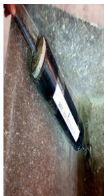
Fig. 10 Grout to sleeve bond failure
