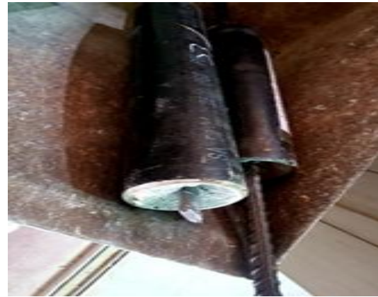
Fig. 11 Bar fracture failure
